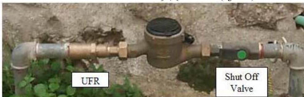
Figure 10: UFR installed, Jerusalem-Ein Karem
